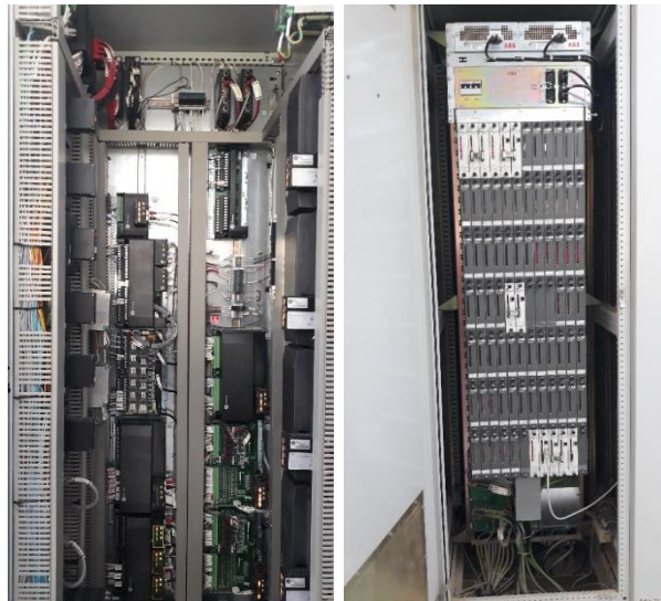
Figure 1.1: Programmable Logic Controller (PLC).
