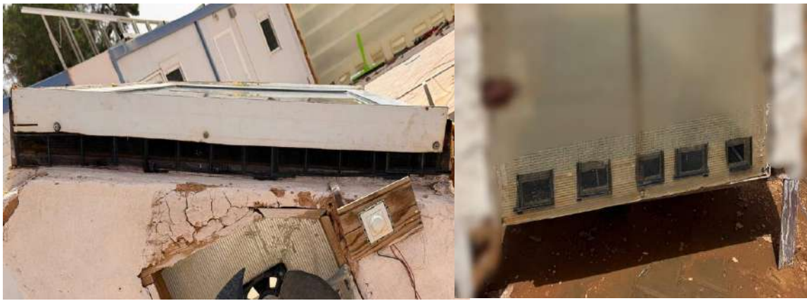
figure.II.13. Air conditioner filters installed in the inlet of Air
