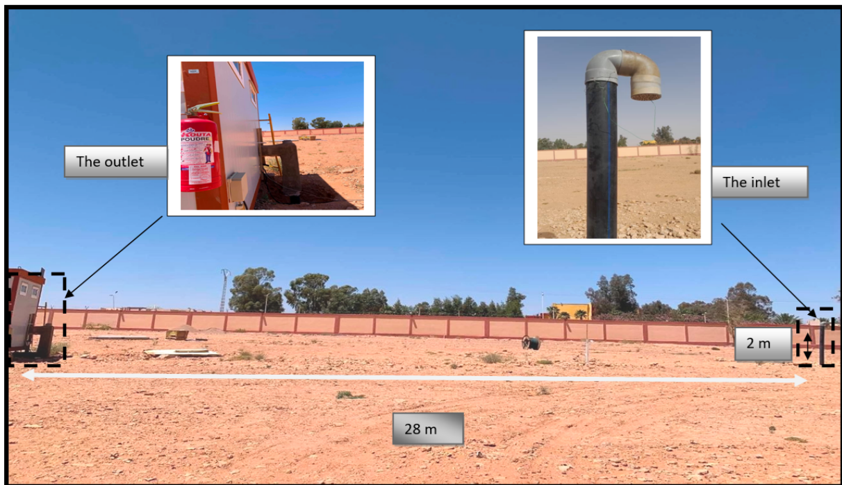
Figure 3-6: Experimental earth-air heat exchanger, URAER (Ghardaïa).
