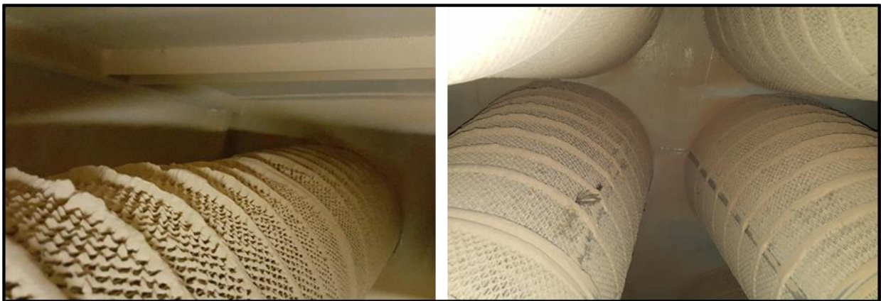
Figure V.9: Condition of air filters
