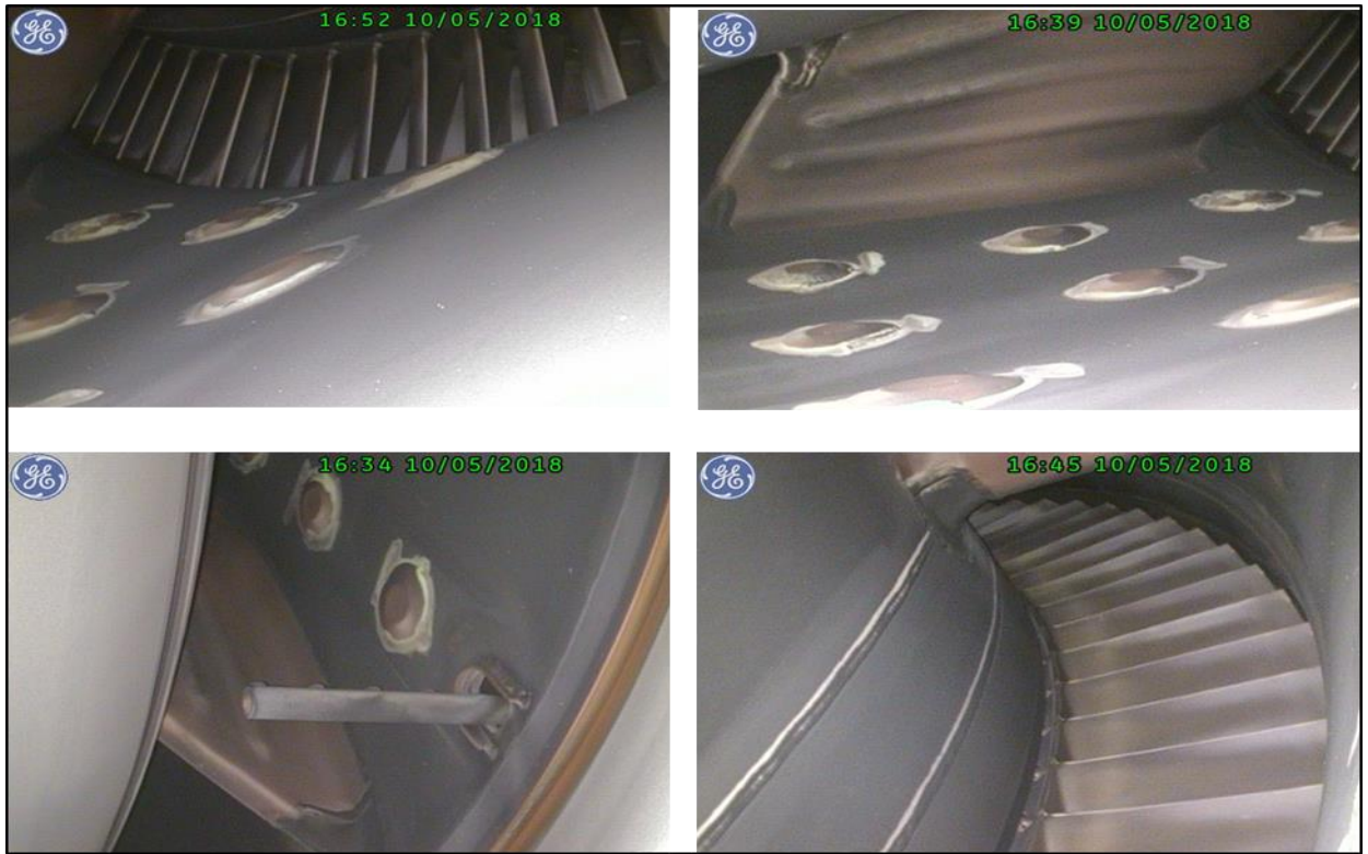
Figure V.7: The interior view with the borescope probe shows that the TMF was in good condition.
