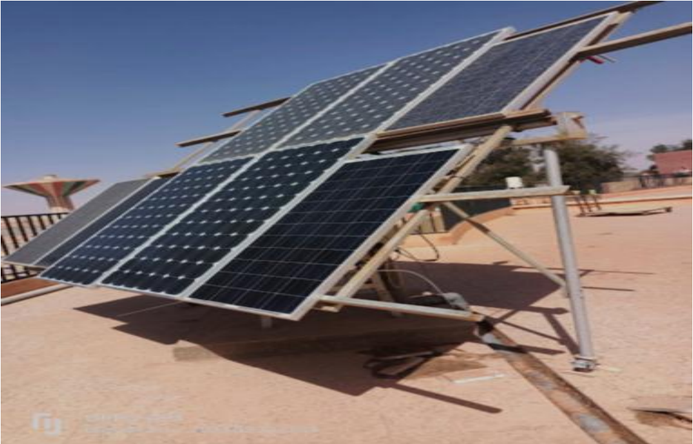
Figure III. 8 SOLO LINE LX - 100M panel photovoltaic installed in URAER.
