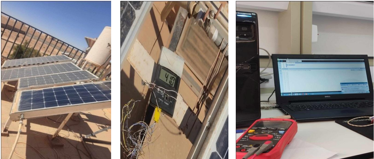
Figure III. 7: SOLO LINE LX - 100M panel photovoltaic installed in URAER used with instruments acquisition.
