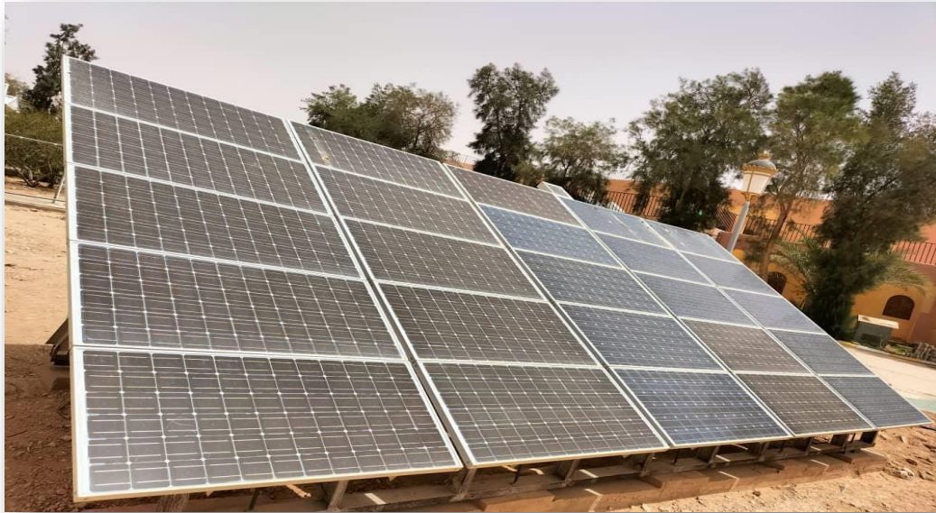
Figure3.7 : PV Generator of ISOFOTON (110W/24V) type.
