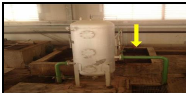
Figure II-21 : Cuve de floculation S-103.[44]
