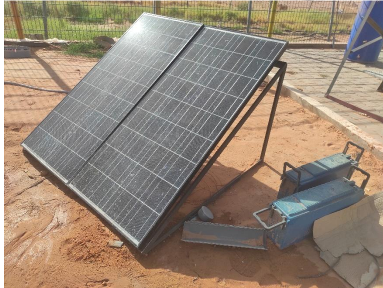
Fig. III. 1. Solar panel 12V.
