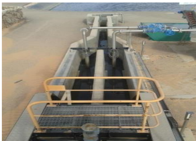
Figure III -3: Dessableur step sidi khouiled.
